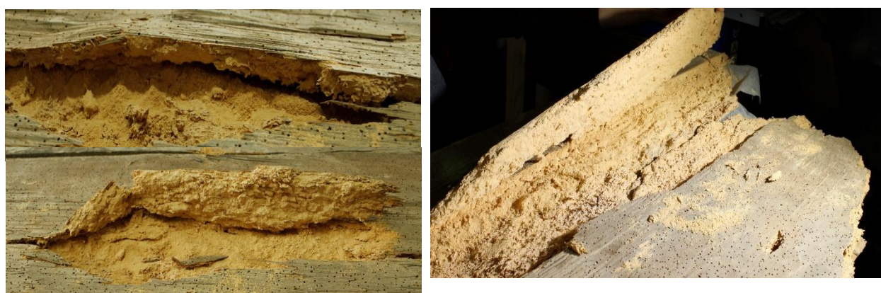
Fig. 2. Severe damage to the wooden support resulting from decimation by wood-eating insects ( original images from the Restoration Laboratory )
